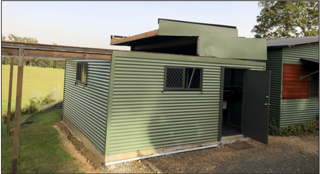
Figure 2. Not how the roof sections should look.
